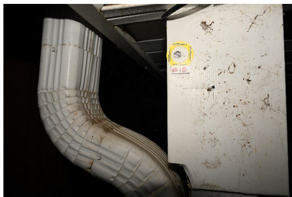
Photos showing approximate view of officers from deck (top); view of defect location in relation to location of officers near shed (middle); and defect in pillar (bottom)
