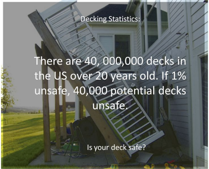
Unsafe connections to beam, ledger.
