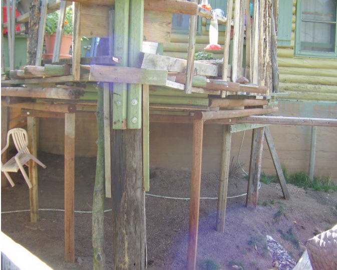
Unsafe deck beams, posts, footings, and rails.
