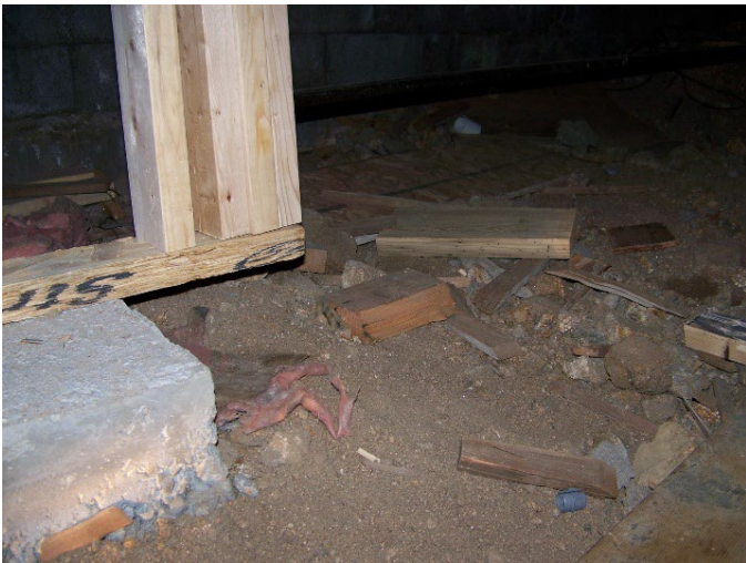
Missing point loads in the crawl space
