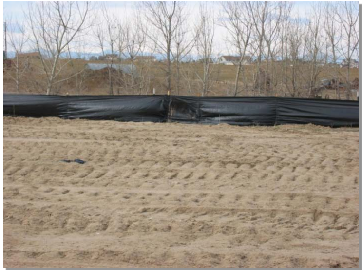
Photograph SF-1. Silt fence creates a sediment barrier, forcing sheet flow runoff to evaporate or infiltrate.
