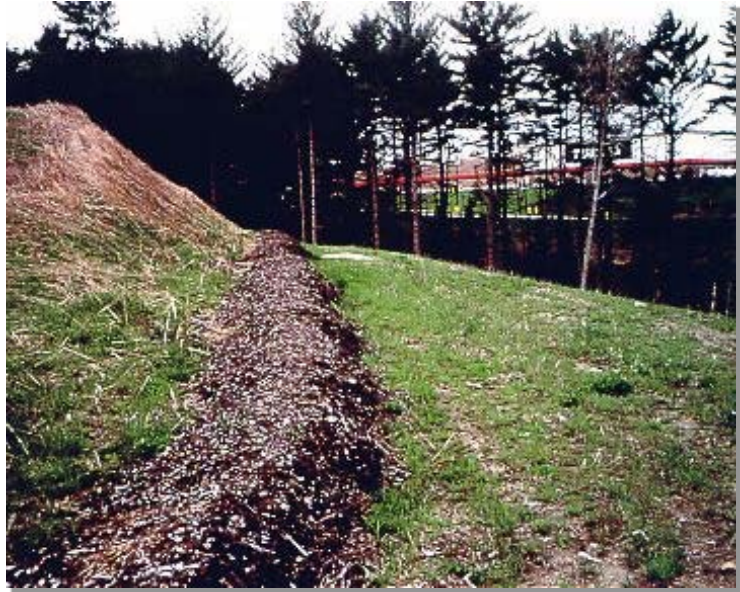
Photograph BB-1. Brush barrier constructed with chipped wood. Photo courtesy of EPA.
