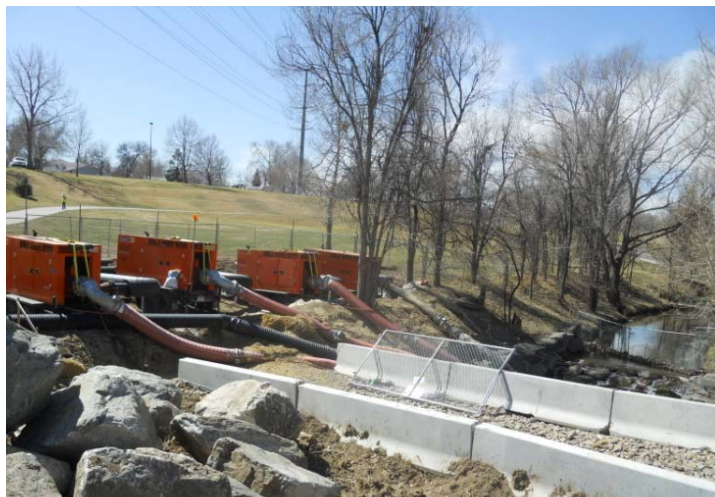
Photograph TDM-2. Despite a relatively significant baseflow, a pumped diversion was selected for this Lakewood Gulch project due to a lack of space crossing Federal Boulevard. Photo courtesy of City and County of Denver.
